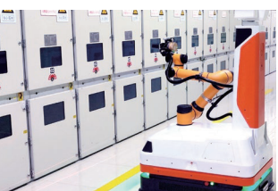
Robotic High-voltage Switchgear Operation
